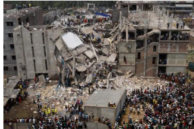
Rana Plaza collapse, Dhaka, Bangladesh, April 24, 2013
